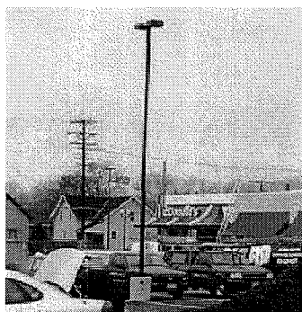
Tall auto oriented lighting fixture
